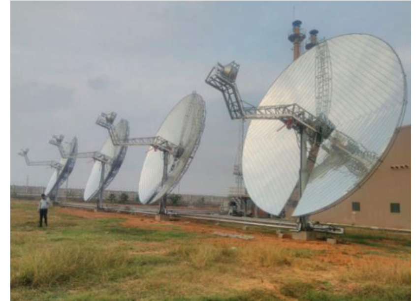
CSH for Cleaning-in-Process at 180 °C employed by confectionery company Mondelez Intl. in India (Source: MWS )
