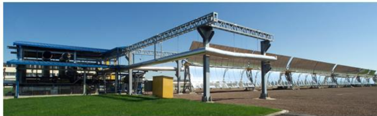
DEMO Sites: Spanish LFC OHLI's pilot plant (Top, left), Atacama LEITAT geosite (Top, right) and Italian PTC ENEA's loop (Bottom)
